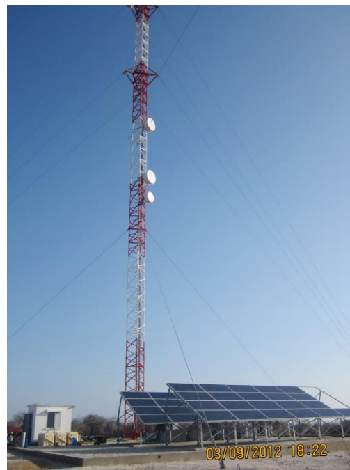
Solar Powered Remote Tower
