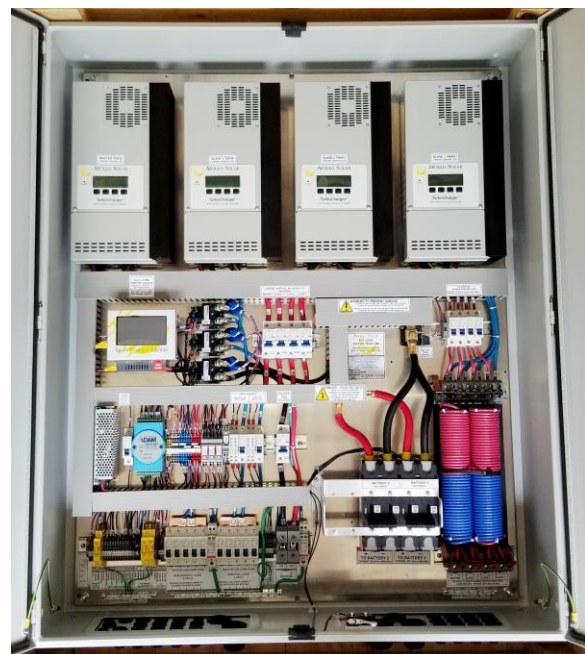
Inside of the Apollo Cabinet for 20kW of PV
