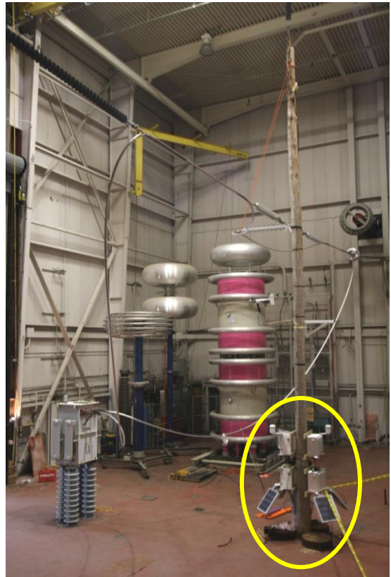
Our equipment taking 25kA strikes
